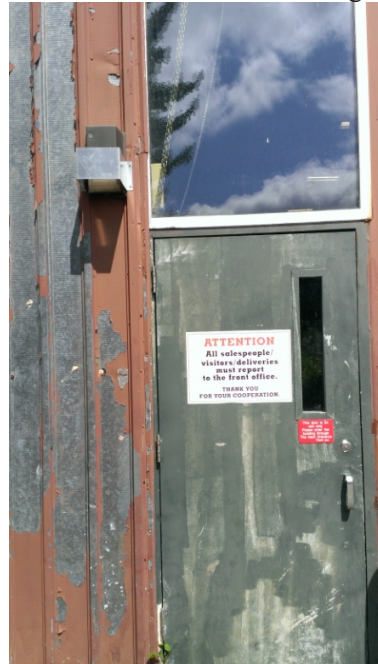
Wall pack with lens covered to reduce glare
