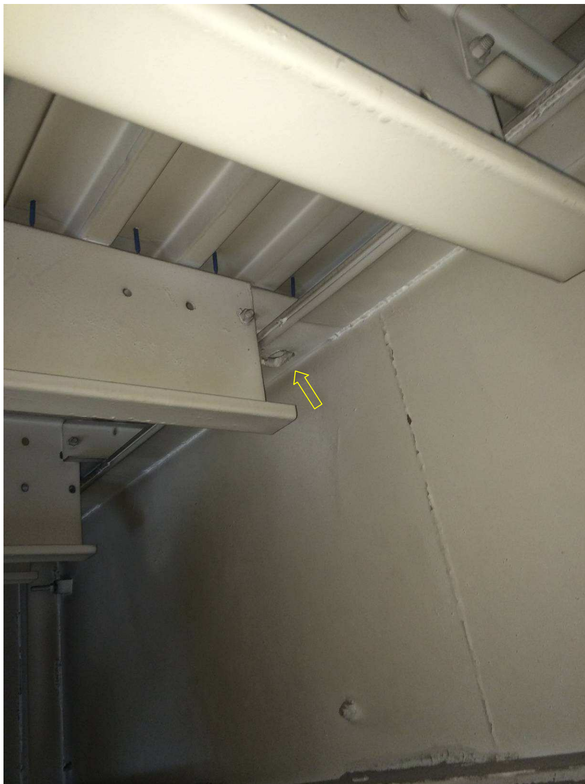
Photo 3: Torched hole in reinforcing plate at beam top flange.
