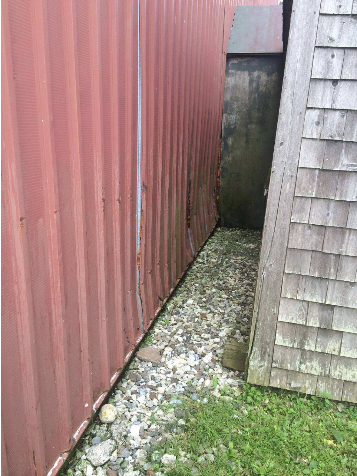
Photo 6: Siding damage and inadequate drainage condition.
