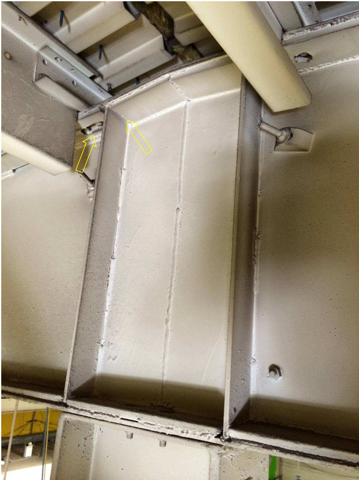
Photo 2: Beam over column connection. Note reinforcing discontinuity at column, holes in top flange reinforcing.
