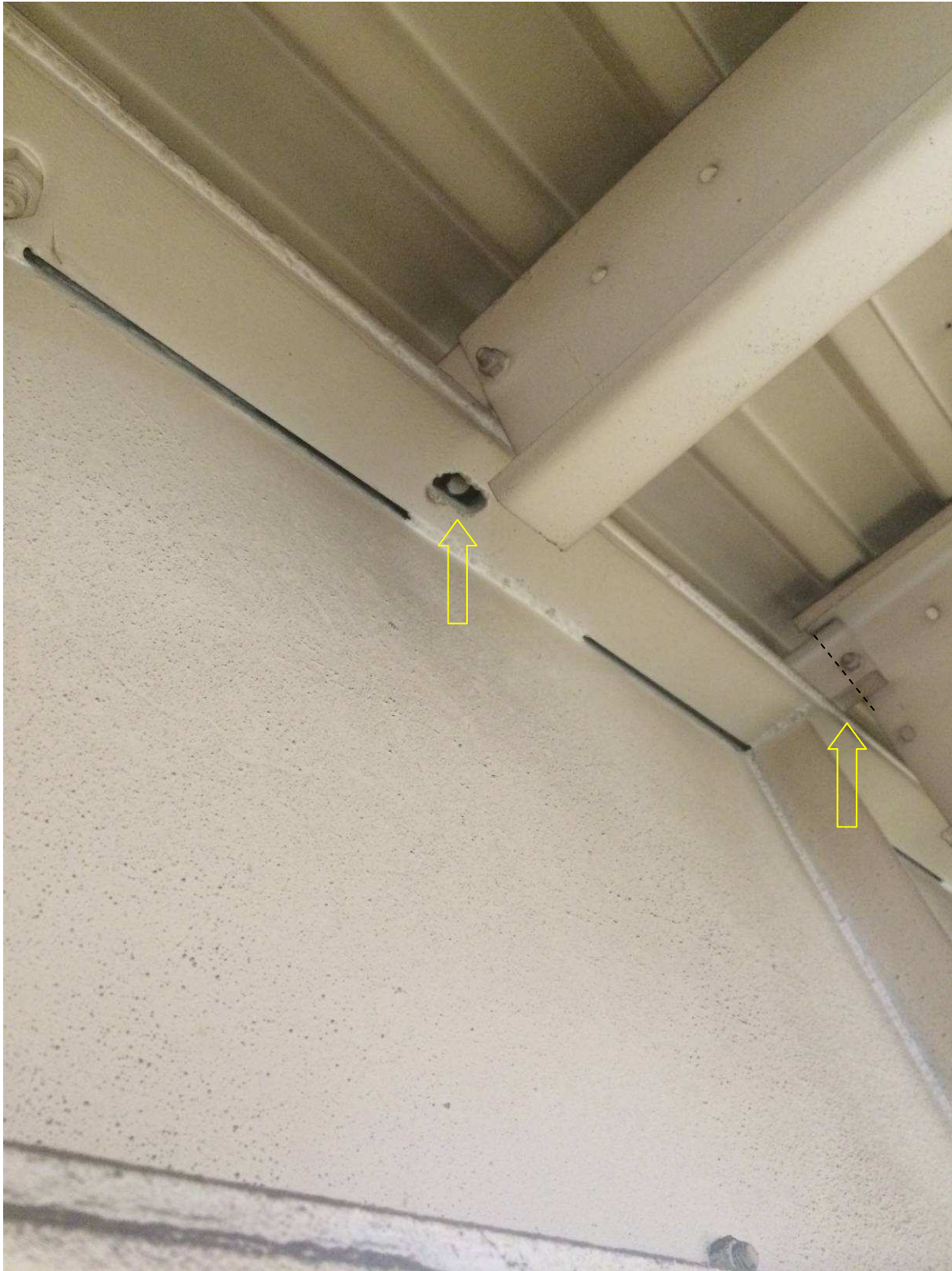
Photo 4: Limited edge distance condition at purlin connection, torched hole in top reinforcing plate.
