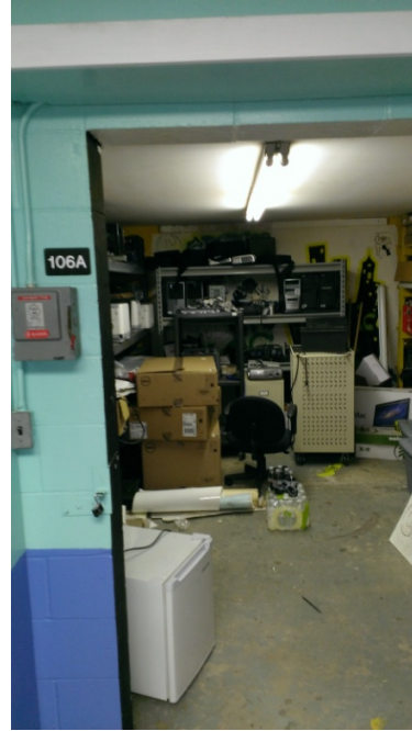
Strip fixture in Storage Room
